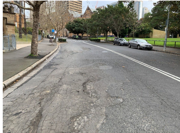
Condition 5 – Very poor
